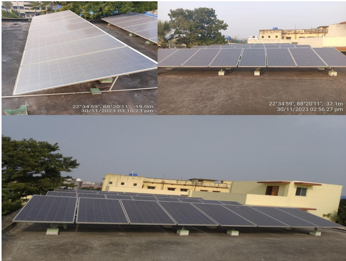
Fig. 7 : Solar Power system for Green Energy
