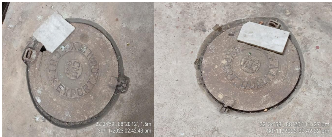
Fig. 6 : Rain water Harvesting Tank
